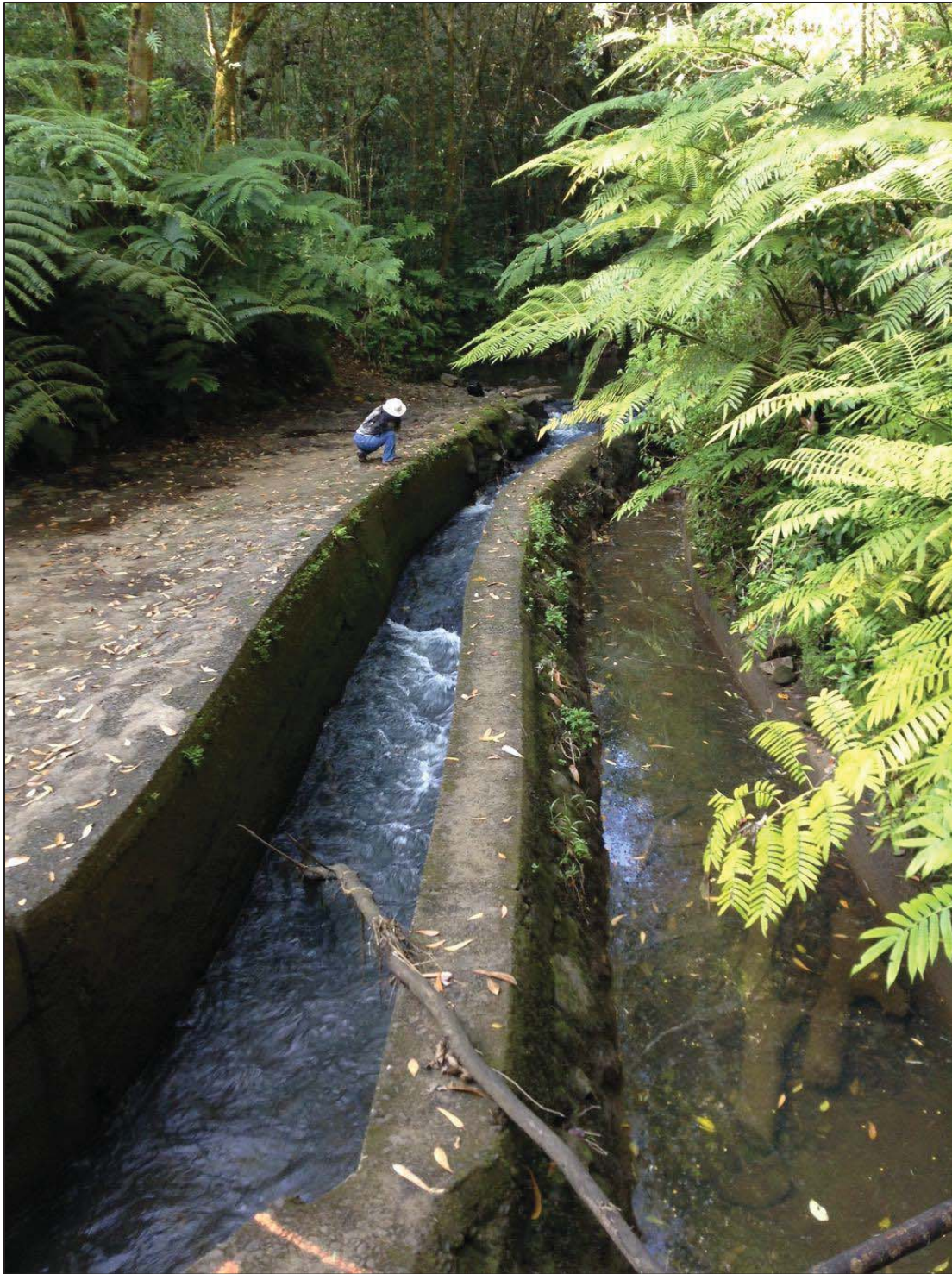
Figure 56. General view of concrete ditches at the Ho'olawali'ili'i sluice gate, view to south
