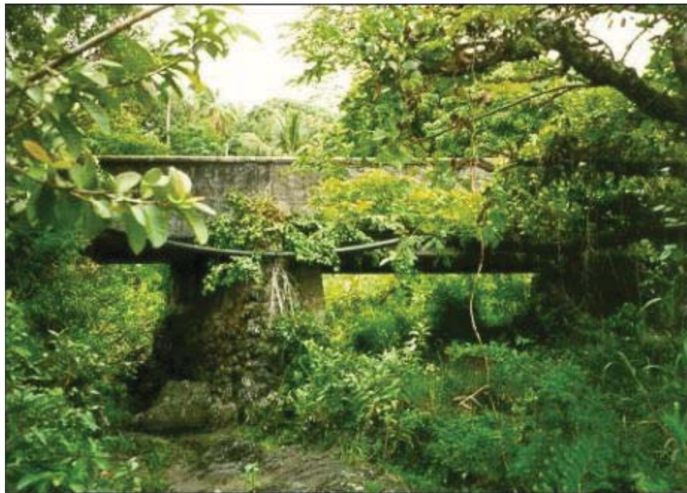
Figure 41. Papahawahawa Stream Bridge, a concrete beam and slab style bridge (Wilson Okamoto & Associates 2001)
