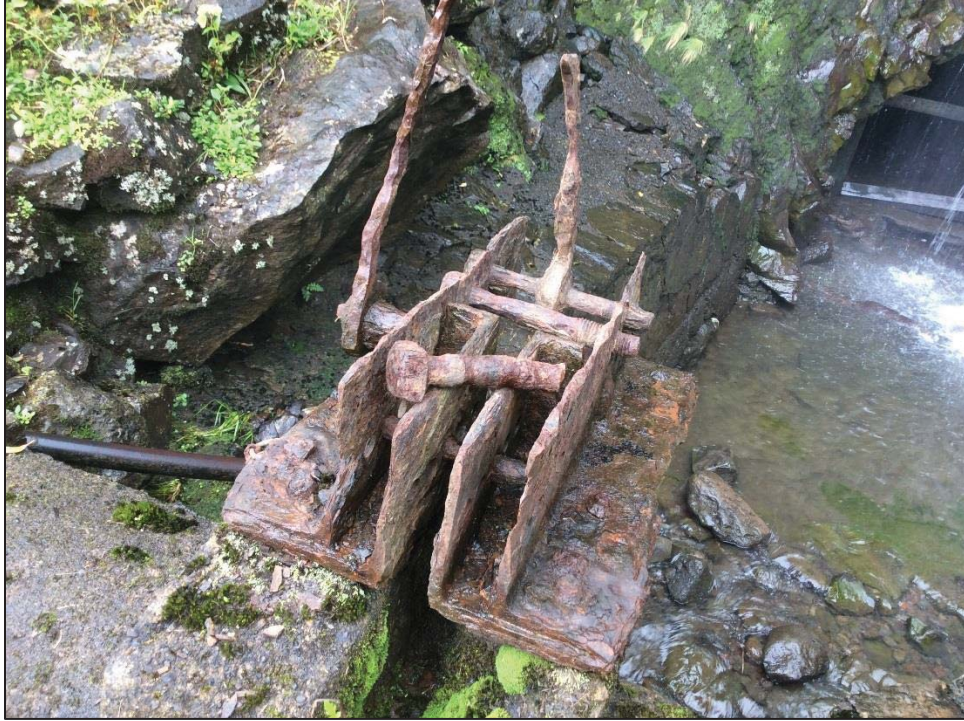
Figure 59. Close-up view of an abandoned iron sluice gate mechanism located along the ditch trail near the Banana sluice gate, view to southeast
