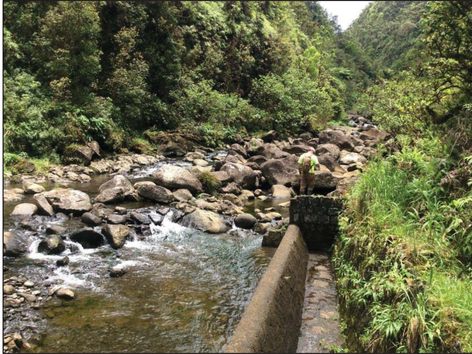
Figure 51. View of archaeologist inspecting the Honomanū Stream bed in the vicinity of the Honomanū sluice gate, view to south
