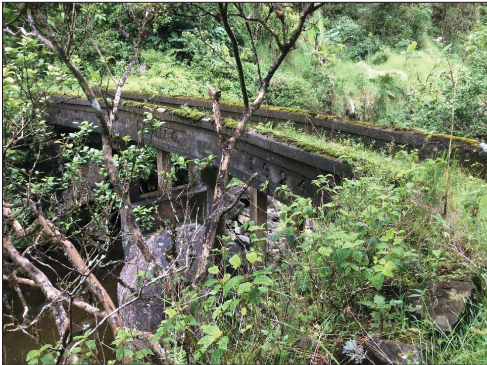
Figure 60. General view of the bridge spanning Honomanū Stream showing “1924” inscribed on side, view to south
