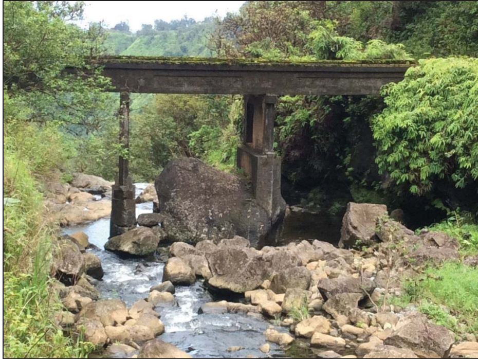
Figure 61. General view of the bridge over Honomanū Stream showing construction that utilizes a massive boulder, view to northeast
