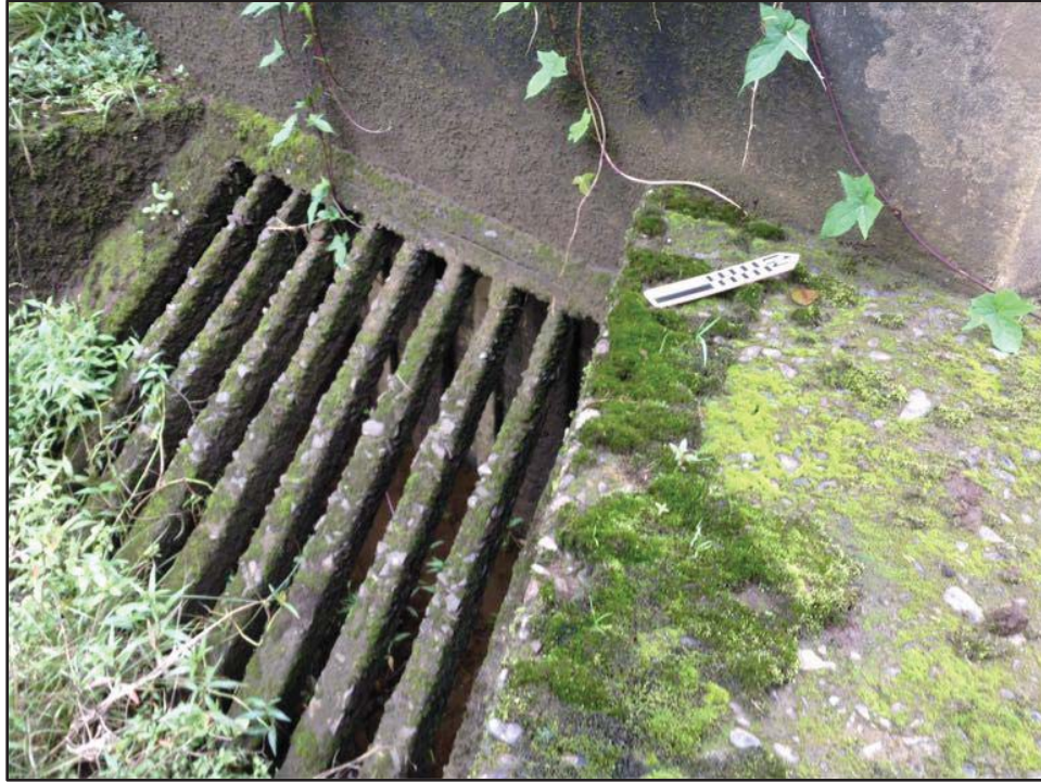
Figure 57. Close-up view of a concrete grate at the East Wailuanui Iki sluice gate, view to west
