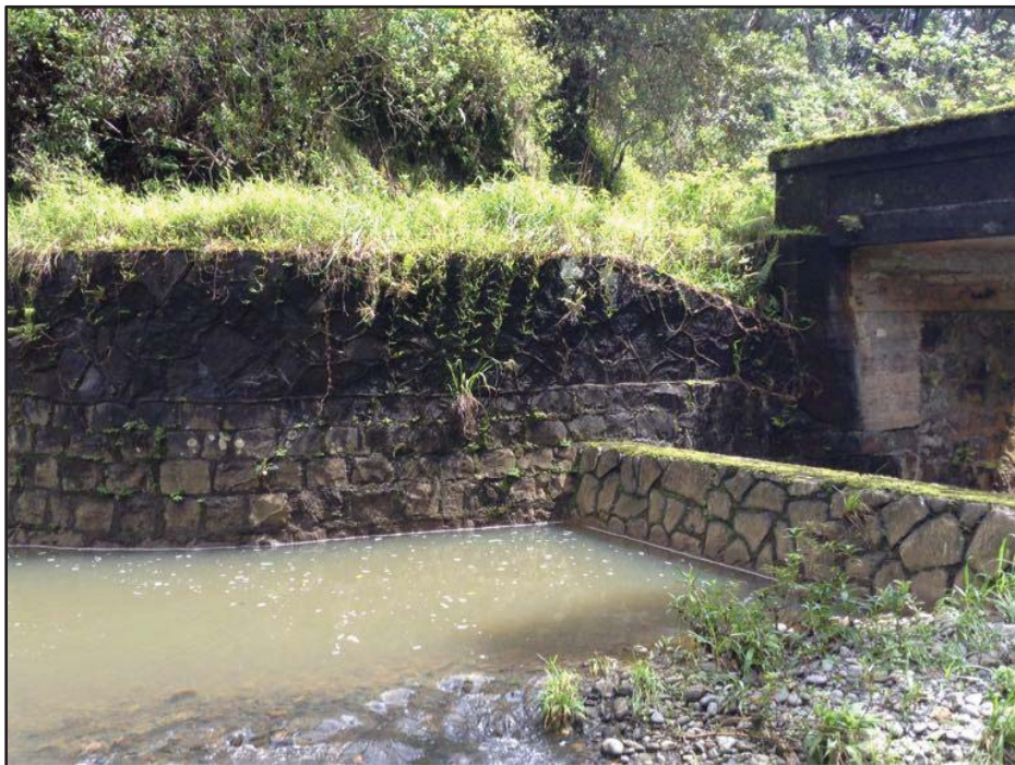
Figure 52. General view of a cut and faced mortared basalt retaining wall located at the West Wailuanui sluice gate, view to northeast
