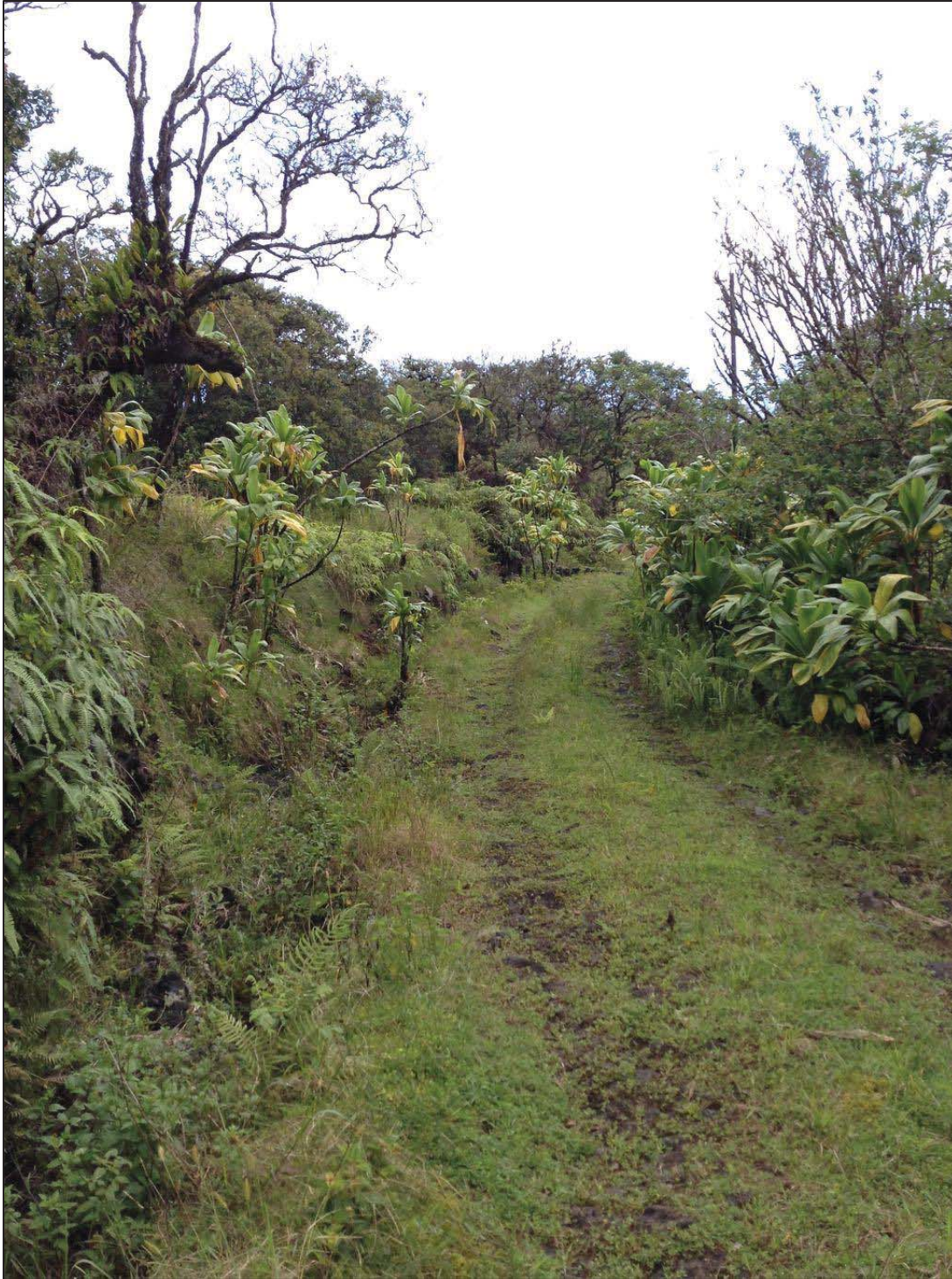
Figure 48. General view of the 4WD access road to the Makapipi sluice gate showing vegetation cover, including large quantities of ti , view to northeast
