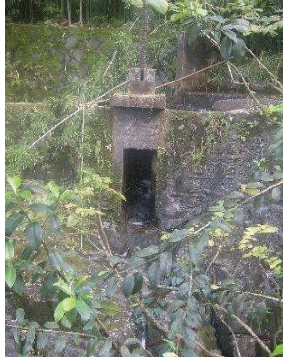
Figure 22: Ratchet sluice gate throw out at Kaaiea stream diversion. Eligible for the Hawaii Register as a contributing feature to a potential district. Integrity largely retained. View facing S. (Source: MAI, 2018)
