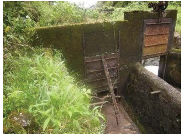
Figure 18: Geared sluice gate at intake at Honomanu stream diversion. Eligible for the Hawaii Register as a contributing feature to a potential district. Integrity largely retained. View facing E. (Source: MAI, 2018)
