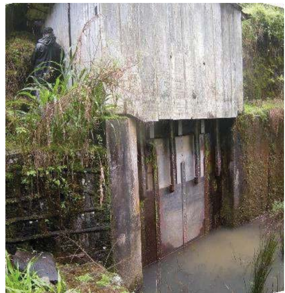
Figure 4: Geared sluice gate at intake at Ko Piliula stream diversion. Eligible for the Hawaii Register as a contributing feature to a potential district. Integrity partially retained. View facing NE. (Source: MAI, 2018)
