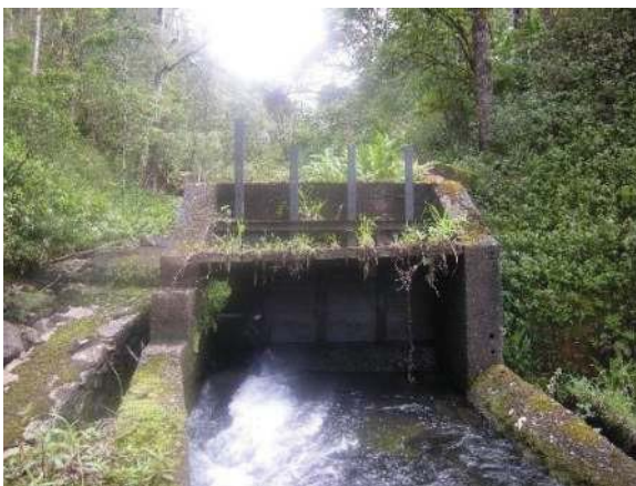
Figure 39: Board adjusted sluice gate at intake of Kolea Power House stream diversion. Eligible for the Hawaii Register as a contributing feature to a potential district. Integrity partially retained. View facing W. (Source: MAI, 2018)
