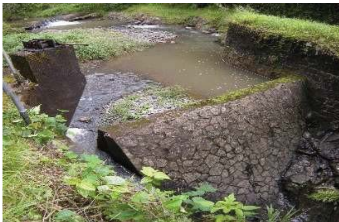
Figure 7: Dam at Wailuanui West Stream diversion impounds stream water for intake. (Source: MAI, 2018)
