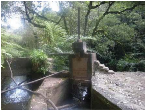
Figure 25: Ratchet sluice gate at Hoolawa Lii Lii stream diversion dam. Eligible for the Hawaii Register as a contributing feature to a potential district. Integrity largely retained. View facing NE. (Source: MAI, 2018)
