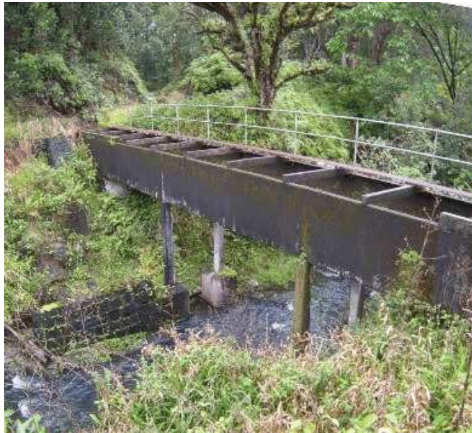
Figure 9: Flume at Koolau Ditch near Waiohue Stream diversion. View Facing N. (Source: MAI, 2018)
