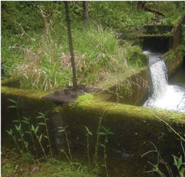
Figure 34: The sluice gate mechanism is a threaded shaft type that is inoperable due to corroded and missing parts. The gate once operated by turning a handwheel that advanced the formerly threaded vertical steel shaft up and down, moving the metal panel. The handwheel is missing and corrosion has destroyed the threads on the steel shaft. Some of these mechanisms have become inoperable due to lack of use. When necessary, however, they can be serviced to make the adjustments. This threaded shaft gate is located at EMI stream diversion at Kolea Power House, on Kolea, a tributary of Punalau, which is ordered to be restored as a “Habitat Stream” by CWRM. View facing S. (Source: MAI, 2018.)
