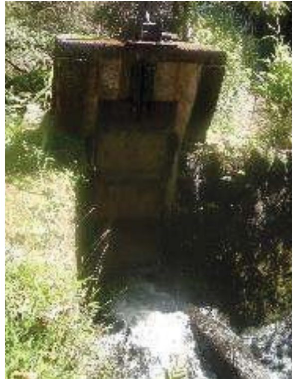
Figure 26: Ratchet sluice gate throw out at intake of Hoolawa Nui stream diversion. Eligible for the Hawaii Register as a contributing feature to a potential district. Integrity largely retained. View facing S. (Source: MAI, 2018)
