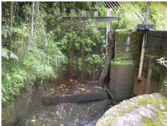
Figure 23: Board adjusted sluice gate (on left) at intake of Hoalua stream diversion. Eligible for the Hawaii Register as a contributing feature to a potential district. Integrity partially retained. View facing NE. (Source: MAI, 2018)
