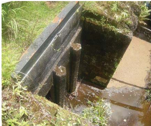
Figure 27: Board adjusted throw out sluice gate at Piinaau throw out. Eligible for the Hawaii Register as a contributing feature to a potential district. Integrity largely retained. View facing NE. (Source: MAI, 2018)
