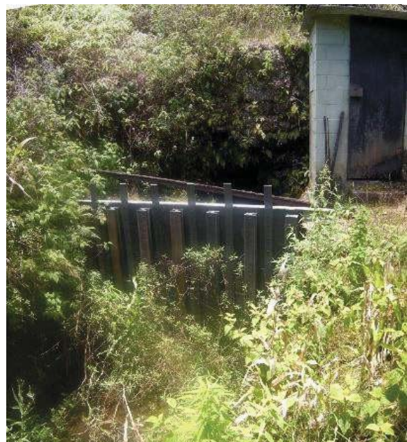
Figure 28: Board adjusted sluice gate at Piinaau throw out. Eligible for the Hawaii Register as a contributing feature to a potential district. Integrity partially retained. View facing SW. (Source: MAI, 2018)
