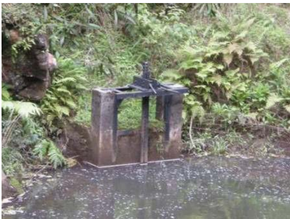
Figure 15: Ratchet sluice gate at intake at Hoolawa Haiku stream diversion. Eligible for the Hawaii Register as a contributing feature to a potential district. Integrity partially retained. View facing E. (Source: MAI)
