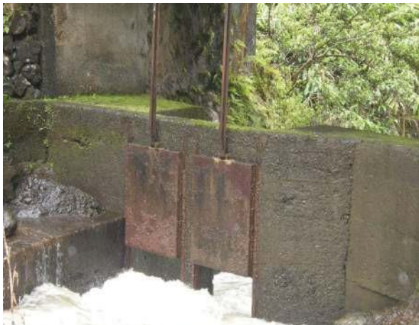
Figure 23: Typical board adjusted type sluice gate mechanism, shown with the gate closed. This gate is located at EMI stream diversion at Waiohue, which is ordered to be a “Fully Restored” stream by CWRM. View facing SE. (Source: MAI, 2018.)
