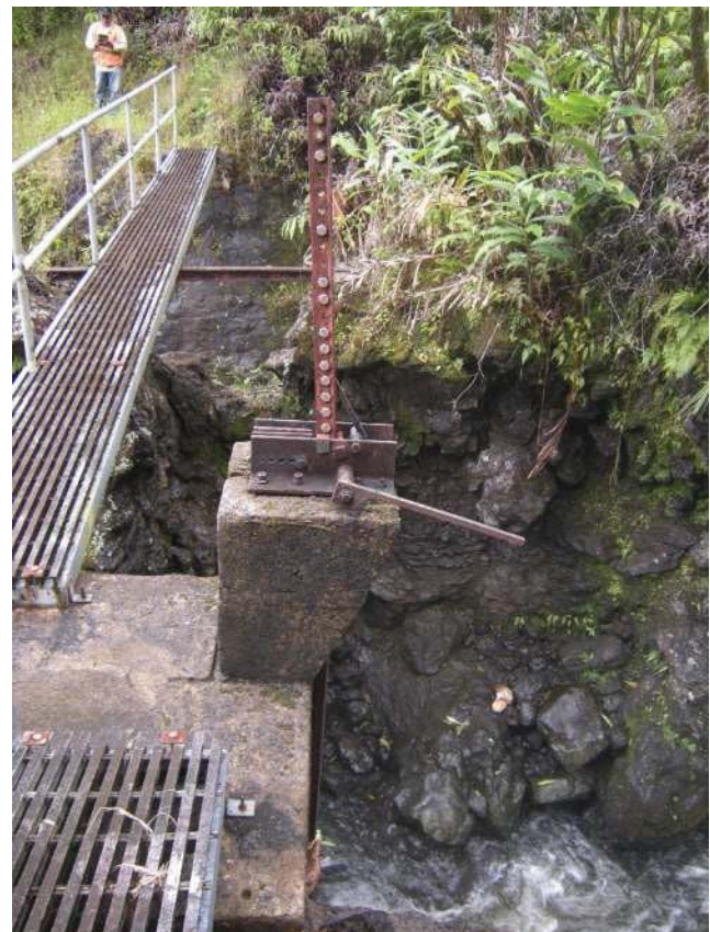
Figure 25: This sluice gate mechanism is a ratchet type. The concrete pedestal and platform it is mounted on is typical of ratchet type gate mechanisms. This ratchet-operating gate is located at EMI stream diversion at Makapipi, which was fully restored in 2008. View facing SE. (Source: MAI, 2018.)
