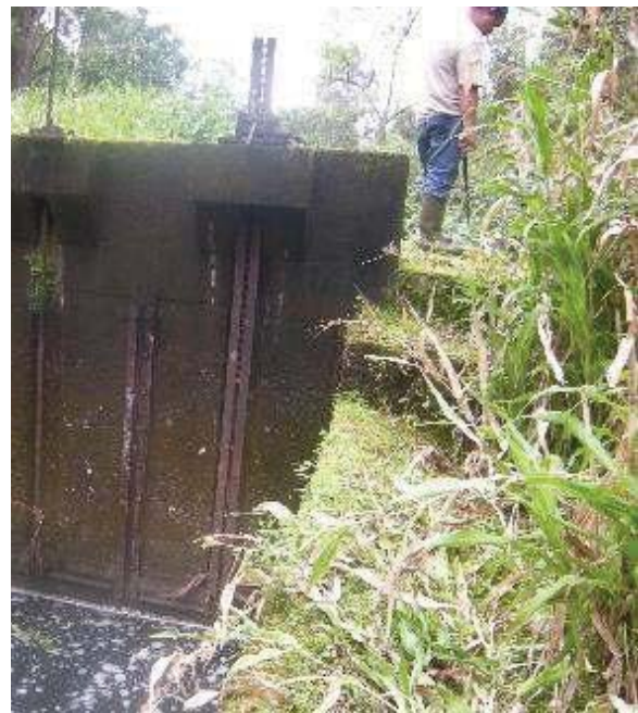
Figure 20: Ratchet sluice gate throw out at intake of Kolea Power House stream diversion. Eligible for the Hawaii Register as a contributing feature to a potential district. Integrity largely retained. View facing N. (Source: MAI, 2018)
