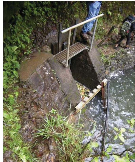
Figure 22: Typical configuration of sluice gates in a concrete dam. These sluice gates are located at EMI stream diversion at Kopiliula, which is ordered to be restored as a “Habitat Stream” by CWRM. View facing N. (Source: MAI, 2018.)
