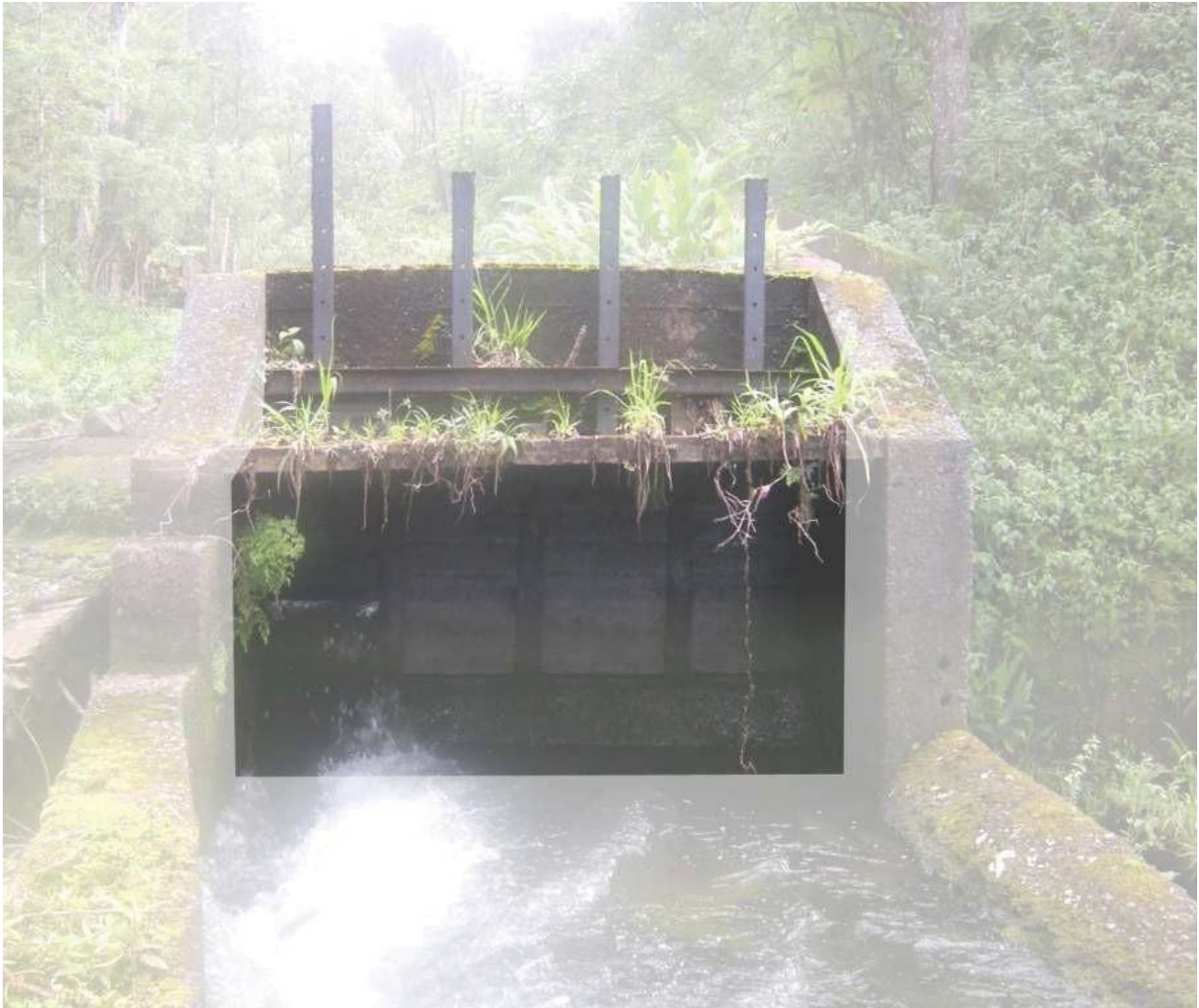
Figure 30: This typical board adjusted type sluice gate operating mechanism is located at EMI Kolea Power House stream diversion on Kolea, a tributary of Punalau, which is ordered to be restored as a “Habitat Stream” by CWRM. View facing SW. (Source: MAI, 2018.)
