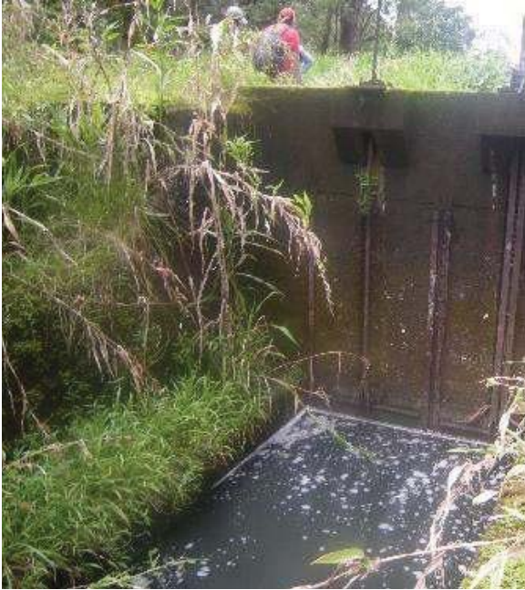
Figure 21: Threaded shaft sluice gate throw out (on left) at intake of Kolea Power House stream diversion. Eligible for the Hawaii Register as a contributing feature to a potential district. Integrity largely retained. View facing N. (Source: MAI, 2018)
