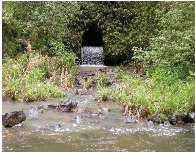
Figure 13: Tunnel near Kopiliula stream diversion carries water underground at ditch gradient. View facing SE. (Source: MAI, 2018.)
