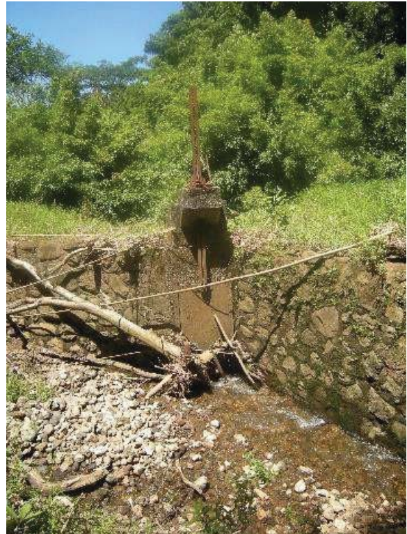
Figure 30: Ratchet sluice gate at Kolea stream diversion dam. Eligible for the Hawaii Register as a contributing feature to a potential district. Integrity largely retained. View facing NE. (Source: MAI, 2018)
