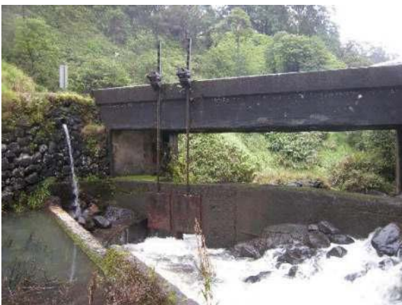
Figure 3: Geared sluice gate at Ko Piliula stream diversion dam. (Two sluice gates shown, side-by-side.) Eligible for the Hawaii Register as a contributing feature to a potential district. Integrity largely retained. View facing N. (Source: MAI, 2018)
