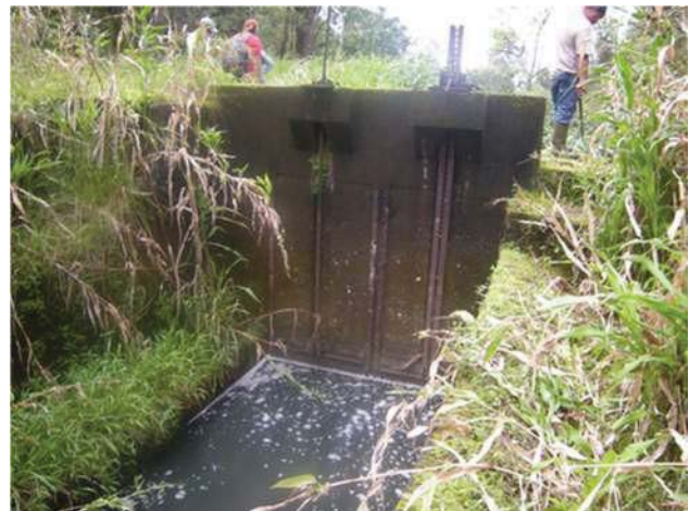
Figure 35: Another view of the threaded shaft gate mechanism at left. This gate is paired with a ratchet type gate. (Source: MAI, 2018.)
