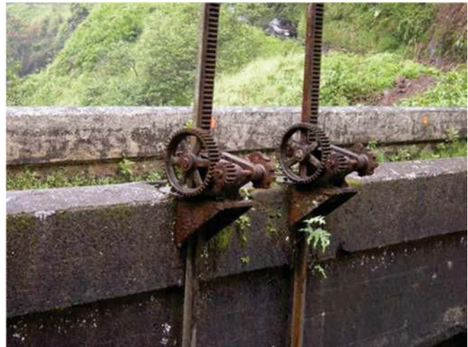
Figure 28: This sluice gate mechanism is a geared type. It operates by attaching a crank to the shaft of the small pinion gear. Revolving the crank operates the geared mechanism and advances the gear rack, to raise or lower the gates. This geared-operating gate is located at EMI stream diversion at Kopiliula, which is ordered to be restored as a “Habitat Stream” by CWRM. View facing E. (Source: MAI, 2018.)
