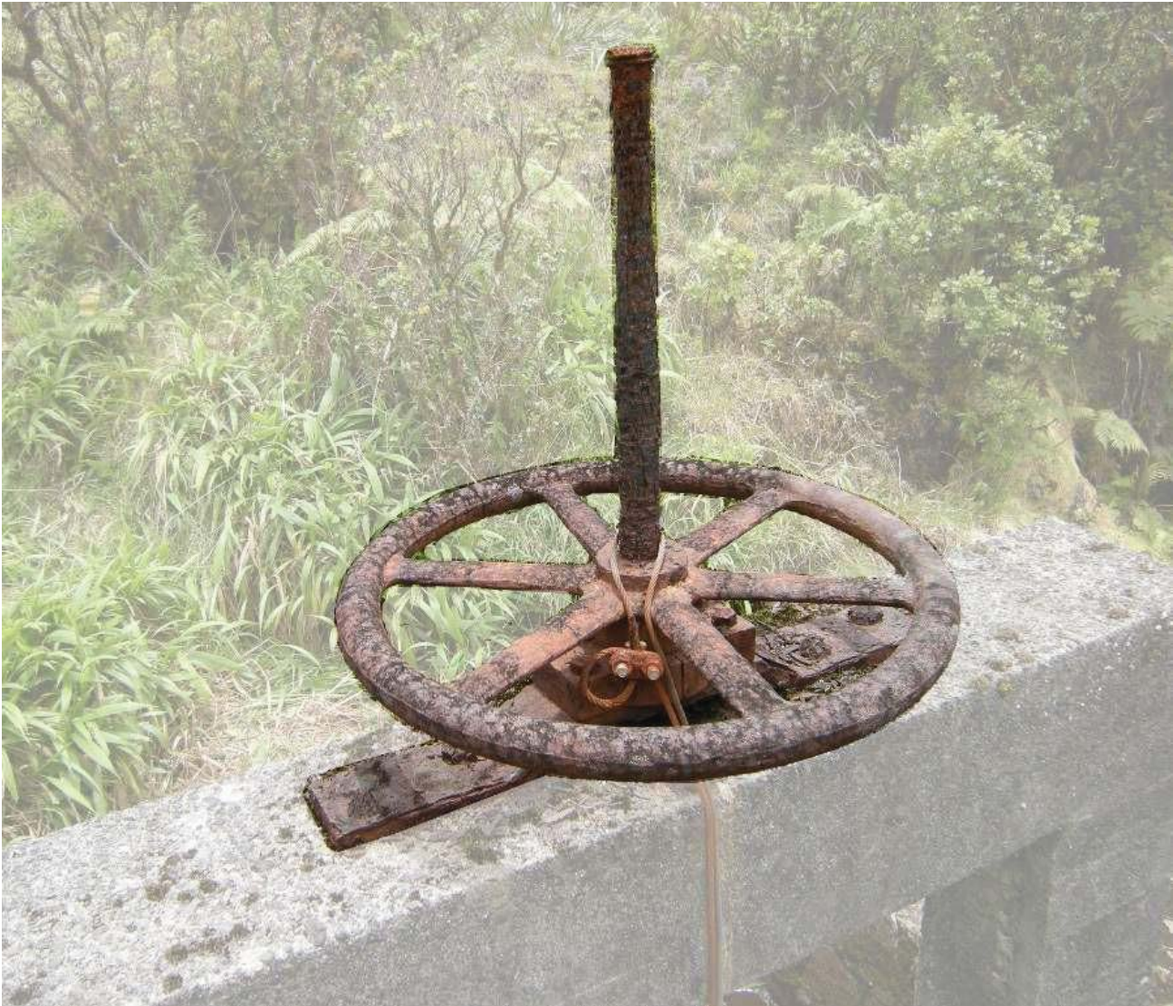
Figure 33: This threaded shaft type sluice gate operating mechanism is located along an irrigation ditch on the Big Island. It is very similar to the threaded shaft mechanism observed at EMI Kolea Power House stream diversion, on Kolea, a tributary of Punalau, which is ordered to be restored as a “Habitat Stream” by CWRM. The single example surveyed was too damaged to properly illustrate its configuration. (Photo: MAI, 2017.)
