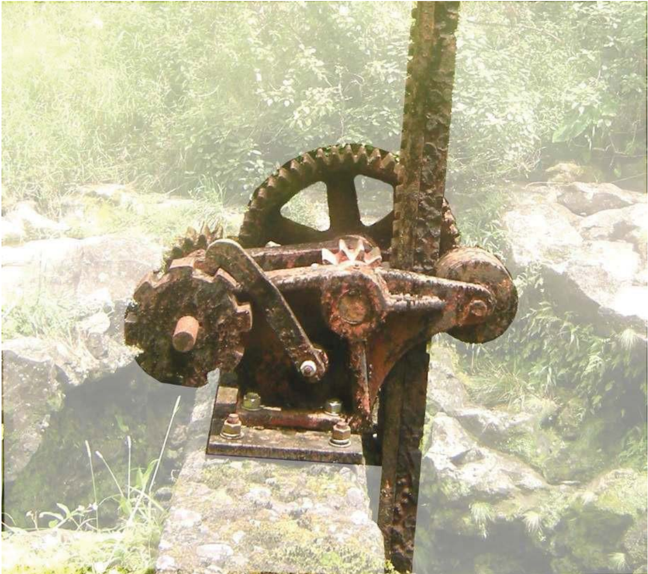
Figure 27: This typical geared type sluice gate operating mechanism is located at EMI Honomanu Stream diversion, which is ordered to be restored as a “Habitat Stream” by CWRM. View facing SE. (Source: MAI, 2018.)
