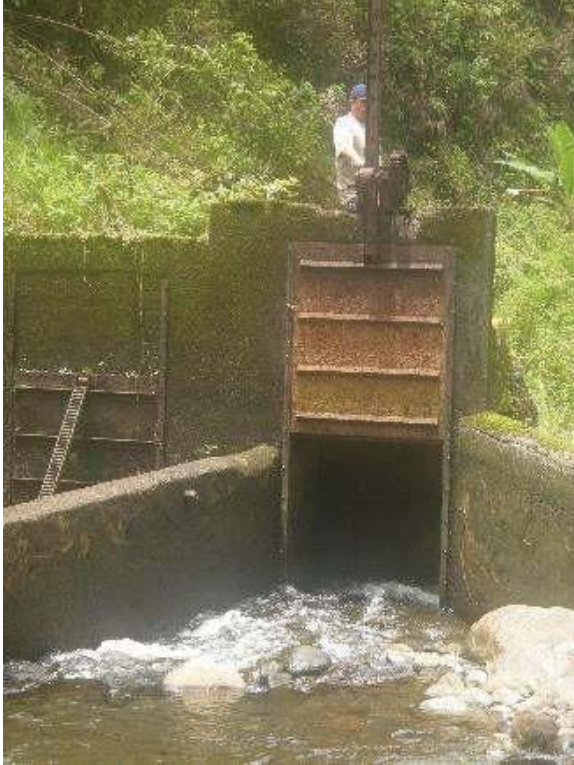
Figure 17: Geared sluice gate at Honomanu stream diversion dam. Eligible for the Hawaii Register as a contributing feature to a potential district. Integrity largely retained. View facing N. (Source: MAI, 2018)
