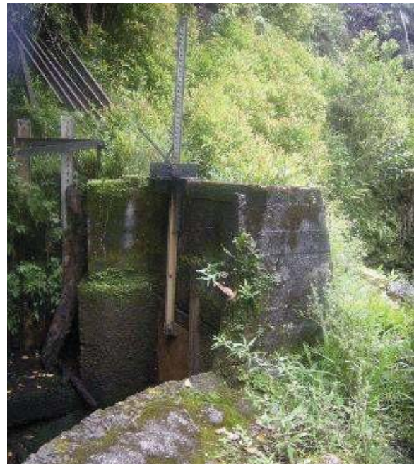
Figure 24: Ratchet sluice gate throw out at intake of Hoalua stream diversion. Eligible for the Hawaii Register as a contributing feature to a potential district. Integrity largely retained. View facing NE. (Source: MAI, 2018)
