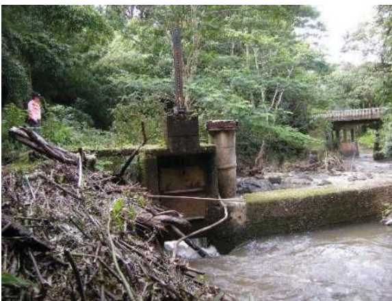
Figure 7: Ratchet sluice gate at Na Ili Ili Haele stream diversion dam. Eligible for the Hawaii Register as a contributing feature to a potential district. Integrity largely retained. View facing NW. (Source: MAI, 2018)
