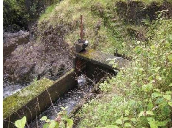
Figure 10: Ratchet sluice gate at Wailua Iki West stream diversion. Eligible for the Hawaii Register as a contributing feature to a potential district. Integrity largely retained. View facing N. (Source: MAI, 2018)
