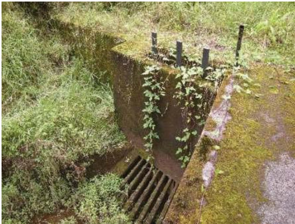
Figure 13: Board adjusted sluice gate at intake of Wailua Iki East stream diversion. Eligible for the Hawaii Register as a contributing feature to a potential district. Integrity partially retained. View facing NW. (Source: MAI, 2018)
