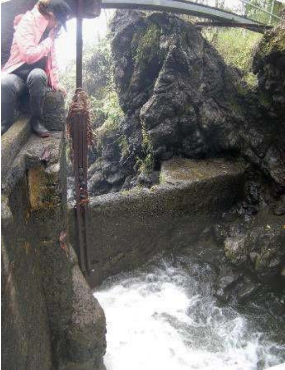
Figure 1: Ratchet sluice gate at Makapipi stream diversion dam. Eligible for the Hawaii Register as a contributing feature to a potential district. Integrity largely retained. View facing SE. (Source: MAI, 2018)
