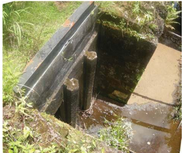
Figure 31: Board adjusted sluice gate with no boards installed. Note that this gate is about 5' wide in total, with three vertical spaces for boards. This board adjusted gate is located at EMI throw-out gate at Piinaau, which is ordered to be a "Fully Restored" stream by CWRM. View facing NE. (Source: MAI, 2018.)
