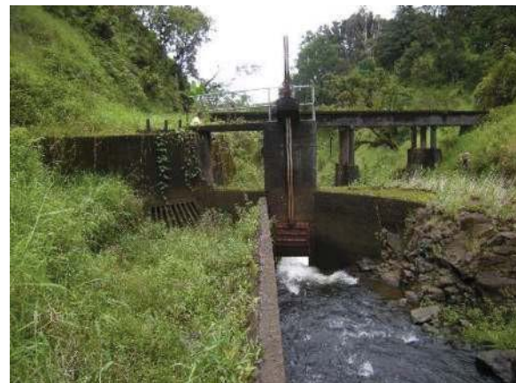
Figure 12: Ratchet sluice gate at Wailua Iki East stream diversion dam. Eligible for the Hawaii Register as a contributing feature to a potential district. Integrity largely retained. View facing NE. (Source: MAI, 2018)
