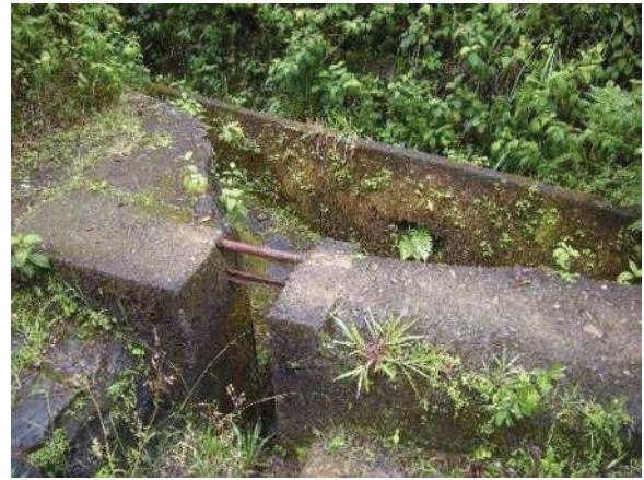
Figure 6: Board adjusted sluice gate throw out at intake of Wai O Hue stream diversion. Eligible for the Hawaii Register as a contributing feature to a potential district. Integrity largely retained. View facing SE. (Source: MAI, 2018)
