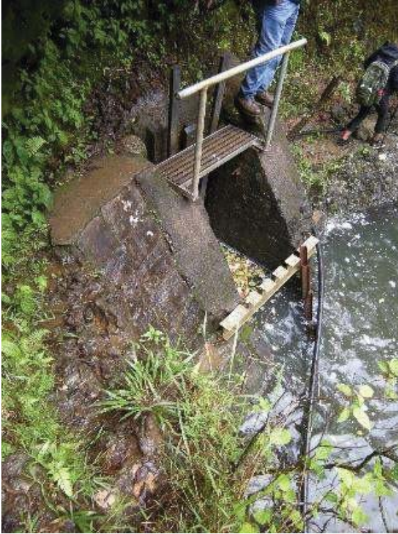
Figure 5: Board adjusted sluice gate at intake of Wai O Hue stream diversion. Eligible for the Hawaii Register as a contributing feature to a potential district. Integrity partially retained. View facing S. (Source: MAI, 2018)
