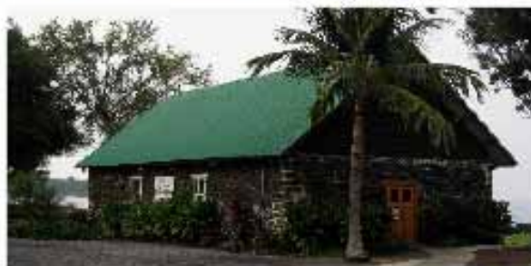
Corrugated red metal roof (above) and Green metal roof accents stone church in Halualoa (below)
